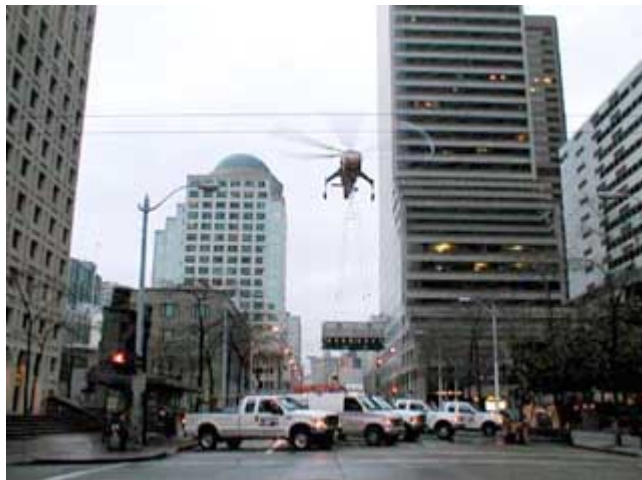
A Sikorsky S-64 "flying crane" lifted the Evapco cooling tower with ease, and placed it atop the Federal Building Feb. 4.
