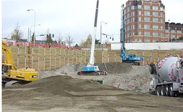
Soldier piles were installed with the help of a track-mounted Watson 3100 drill rig.
