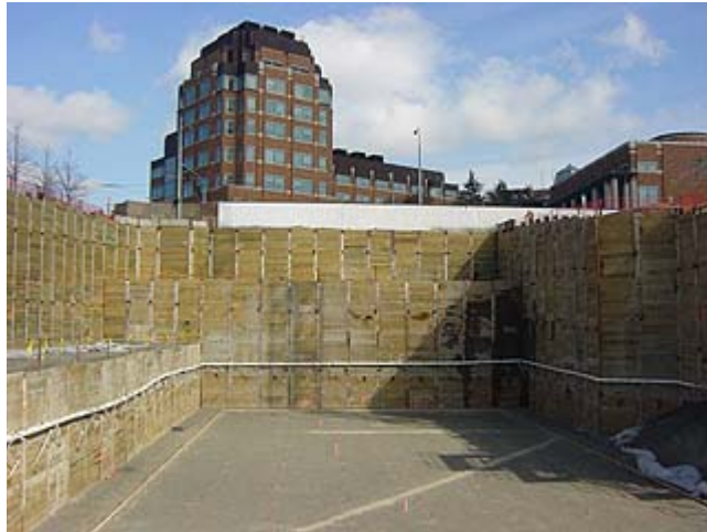
Photos courtesy of Malcolm Drilling Co. Excavation depths reached 55 feet at the north end of the hole for the UW Bioengineering-Genome Sciences Building.
